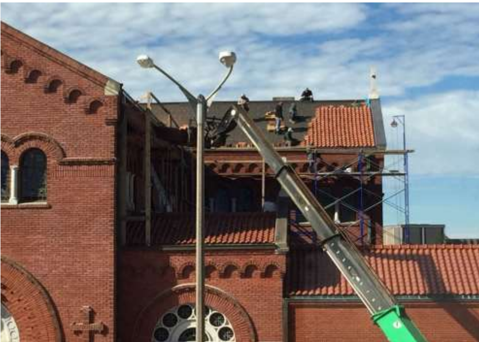
The outside HVAC units are in place, and now working on the mechanical yard enclosure.
