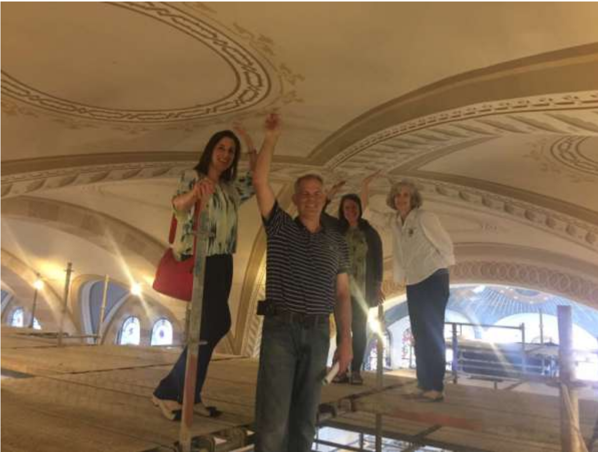
Some even ventured to the top of the scaffolding for a rare opportunity to touch the ceiling!
