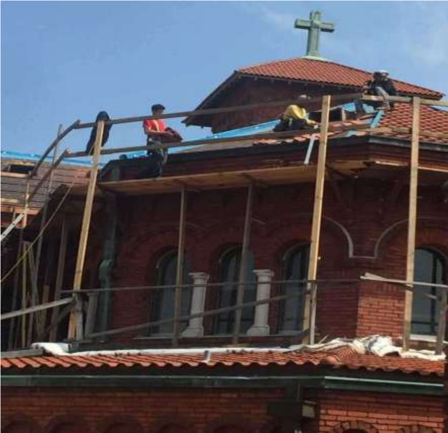
Roofers from Ribbeck Construction working on the roofs above the altar and apse.
