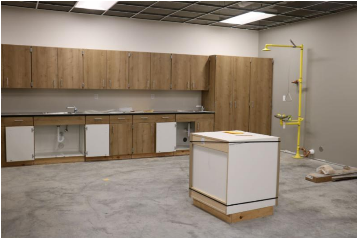
The interior work continues in the main Academic Center. This view looks toward the library.
